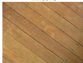
Figure 26. Wooden floor showing existing gaps
