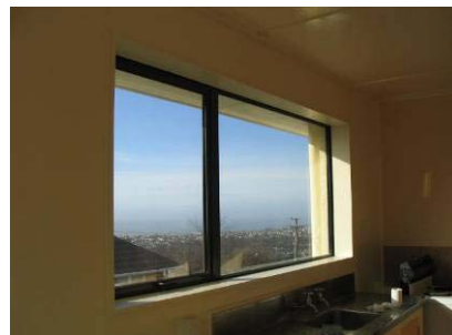
Figure 14. New double glazed aluminium framed windows.
