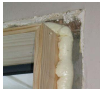
Figure 25. Foam around window seal in new windows
