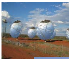
Solar System's 220 kWp concentrator system (Pitjantjatjara, SA)
