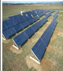
EnergyAustralia's Singleton PV power station
